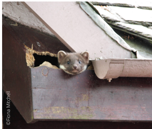
Damage to timber roofing structure creating an access point.
