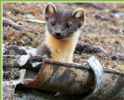
Examples of damaged roofs through which pine martens can access loft spaces.
