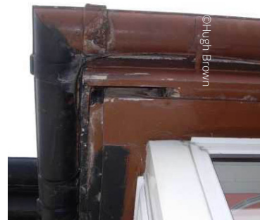
Soffit with a potential access point for pine martens.
