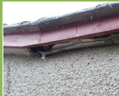
Examples of damaged soffits through which pine martens can access loft spaces.
